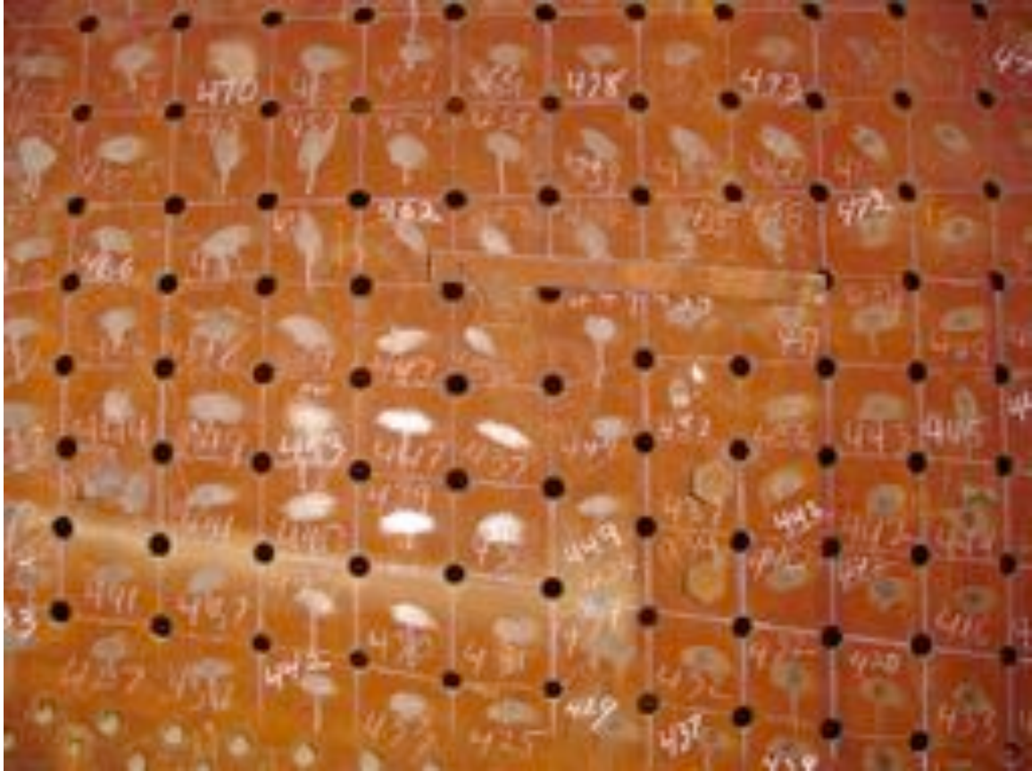
In this photo of 39's side sheets, note the polished metal evenly spaced between each staybolt hole. It is here that the UT readings are taken. The number is the thickness reading found at that location.
